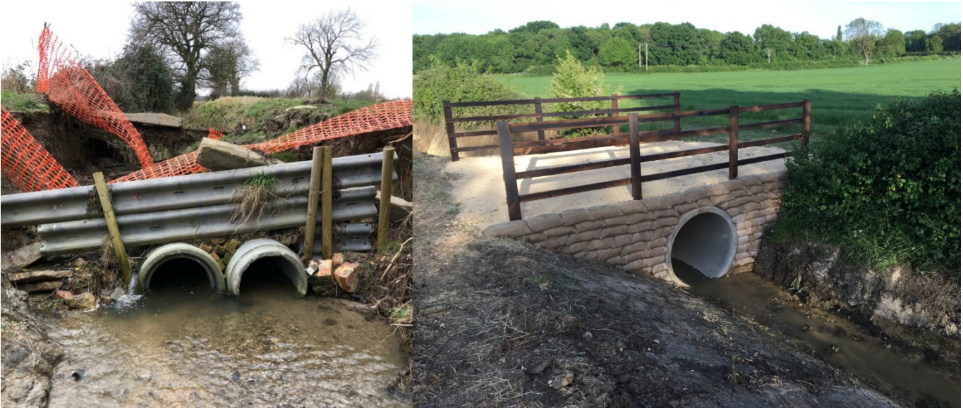
Figure 7-3 Culvert collapse and subsequent on Marholm Brook
