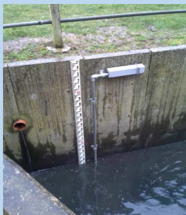
Figure 7-4 Water level monitoring installation in Peterborough
