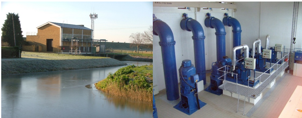
Figures 5-10 and 5-11: Cross Guns Pumping Station inside (left) and outside (right). Source: North Level District IDB
